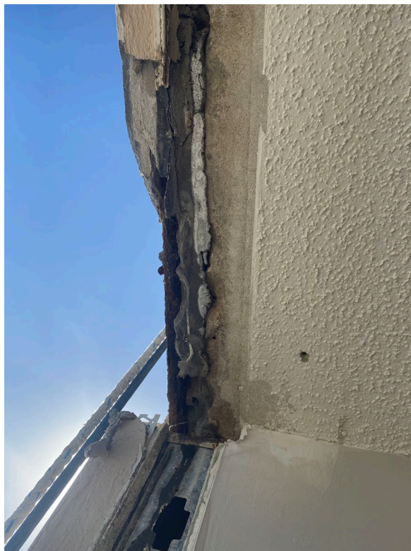
Picture 3: Unit 507 header spall
