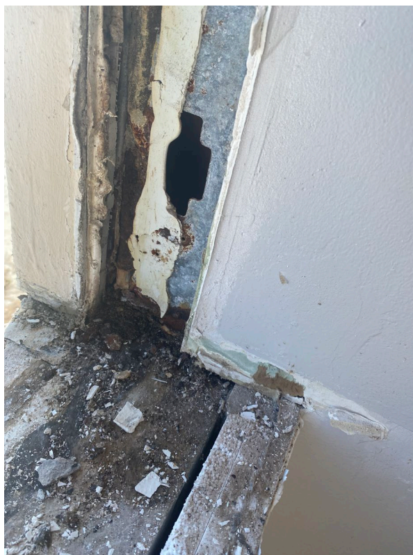
Picture 4: Unit 507 South jamb corrosion
